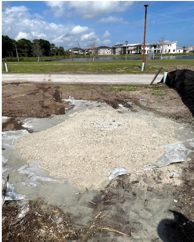
Figure 7-3. Concrete washout disposed directly on a tarp on the ground.
