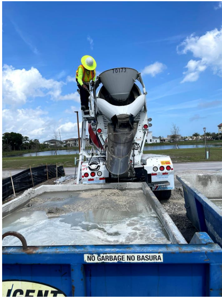
Figure 4-1. Concrete washout placed in specific fabricated container which will be collected and recycled.
