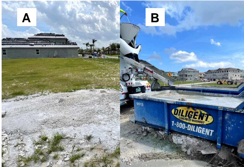
Figure ES-1. Concrete being washout out: A) directly on the ground which is the worst management collection approach and; B) into a best management collection container which will be transported with about 100% clean concrete washout that will be recycled/reused by crushing or as a lake fill material.
