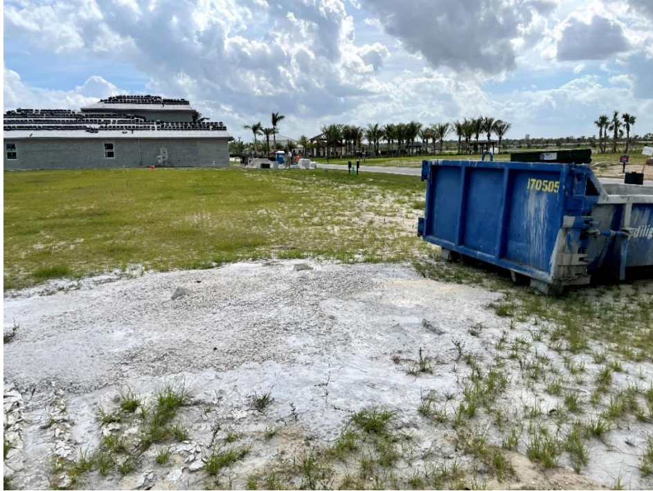
Figure 7-2. Concrete washout placed directly on ground; this is the worst management collection approach.
